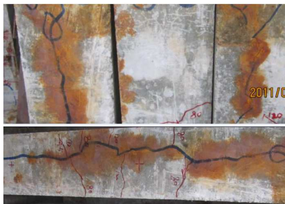
Fig. 6. Corrosion crack map and bending load crack
