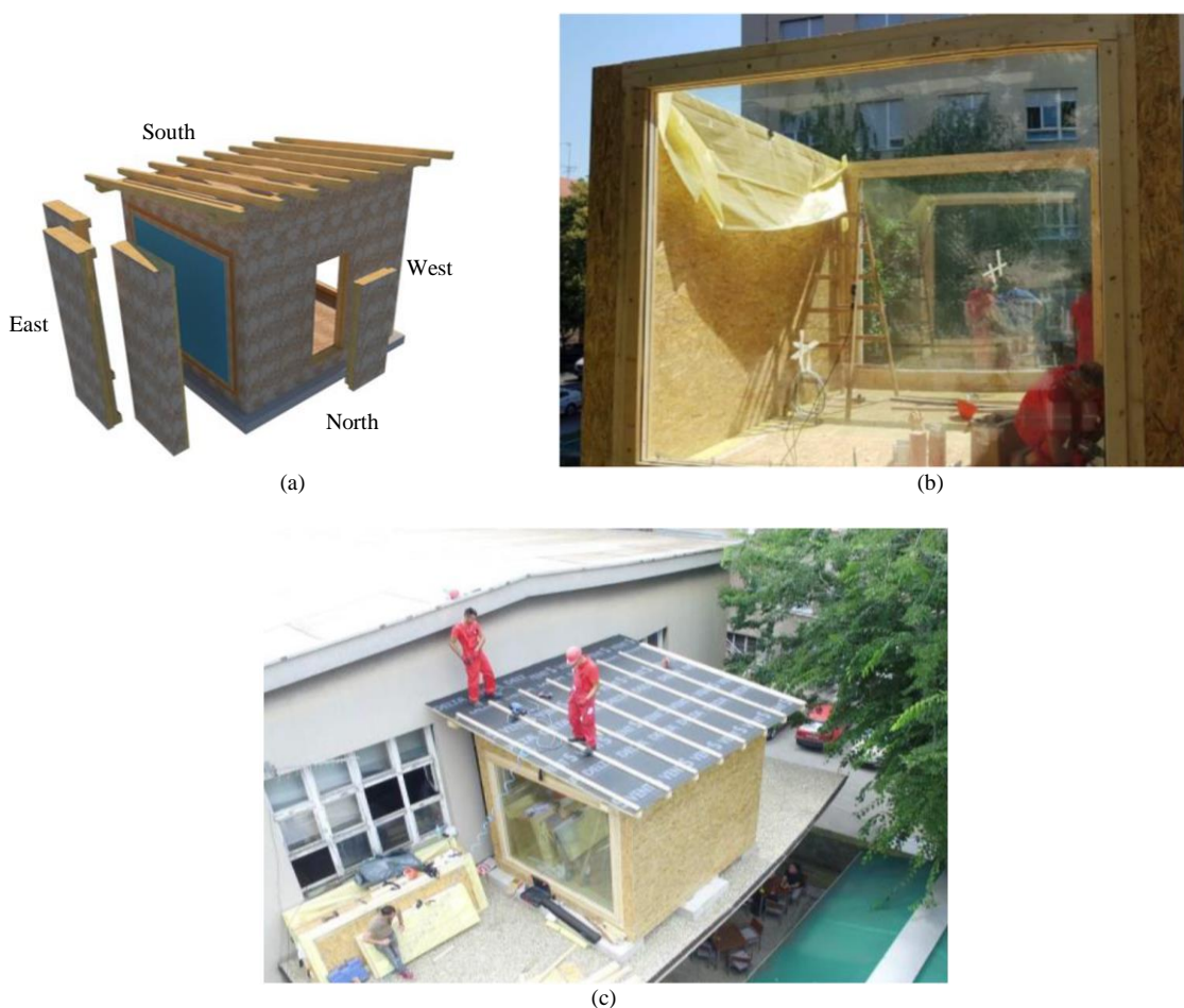
Fig. 6: Assembly process for the Live-Lab facility at the University of Zagreb, Croatia (installation during 2018): (a) general concept; (b) CLT-glass facade elements and (c) roof
