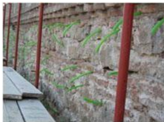
Fig. 9: Grouting-the installment of the grout through rubber tubes in the wall (Christou and Elliotis, 2016)
